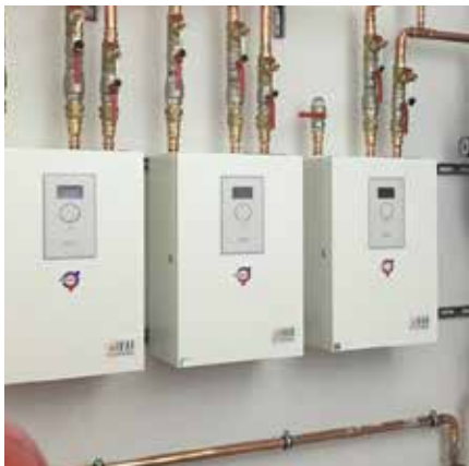
Atec control system (indoor)
